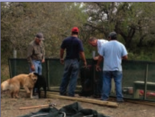
Thomas Moore Feed Co. personnel building the blind, and water features at Thomas' Meadow; sign by LMN.
