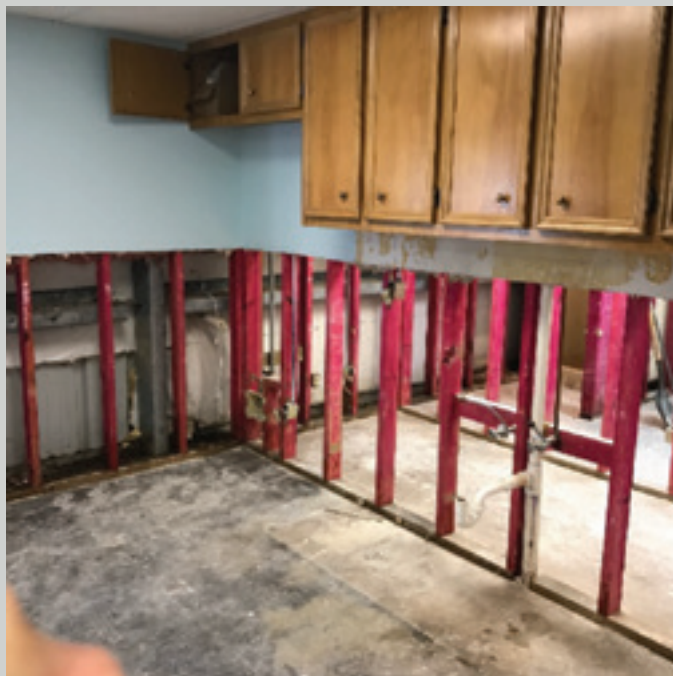
The GCBO Field House was totally gutted after flood waters. Photo Credit: Martin Hagne.
