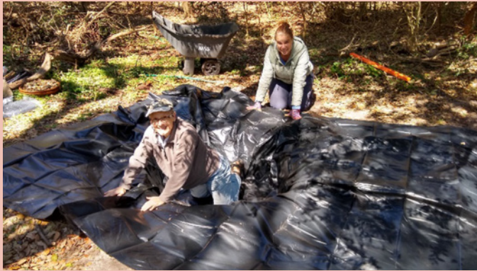
After the hard work is done, then comes the liner. Shelia Hargis pitches in to help with this part, with Kendra overseeing her work. Photo credit: James Giroux
